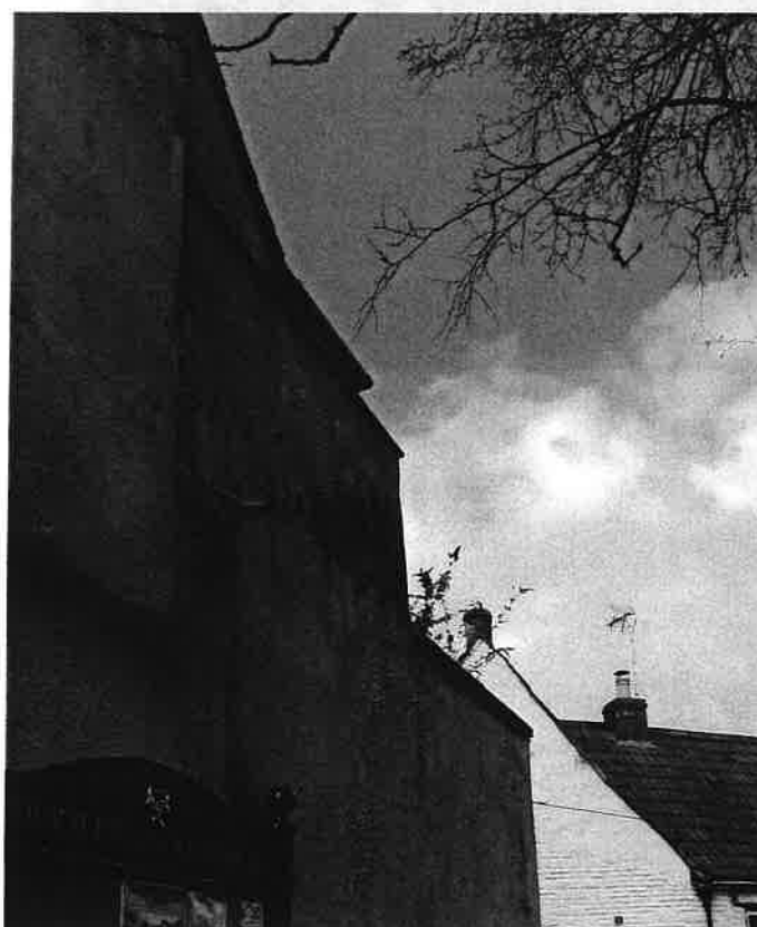
Plants growing in guttering
