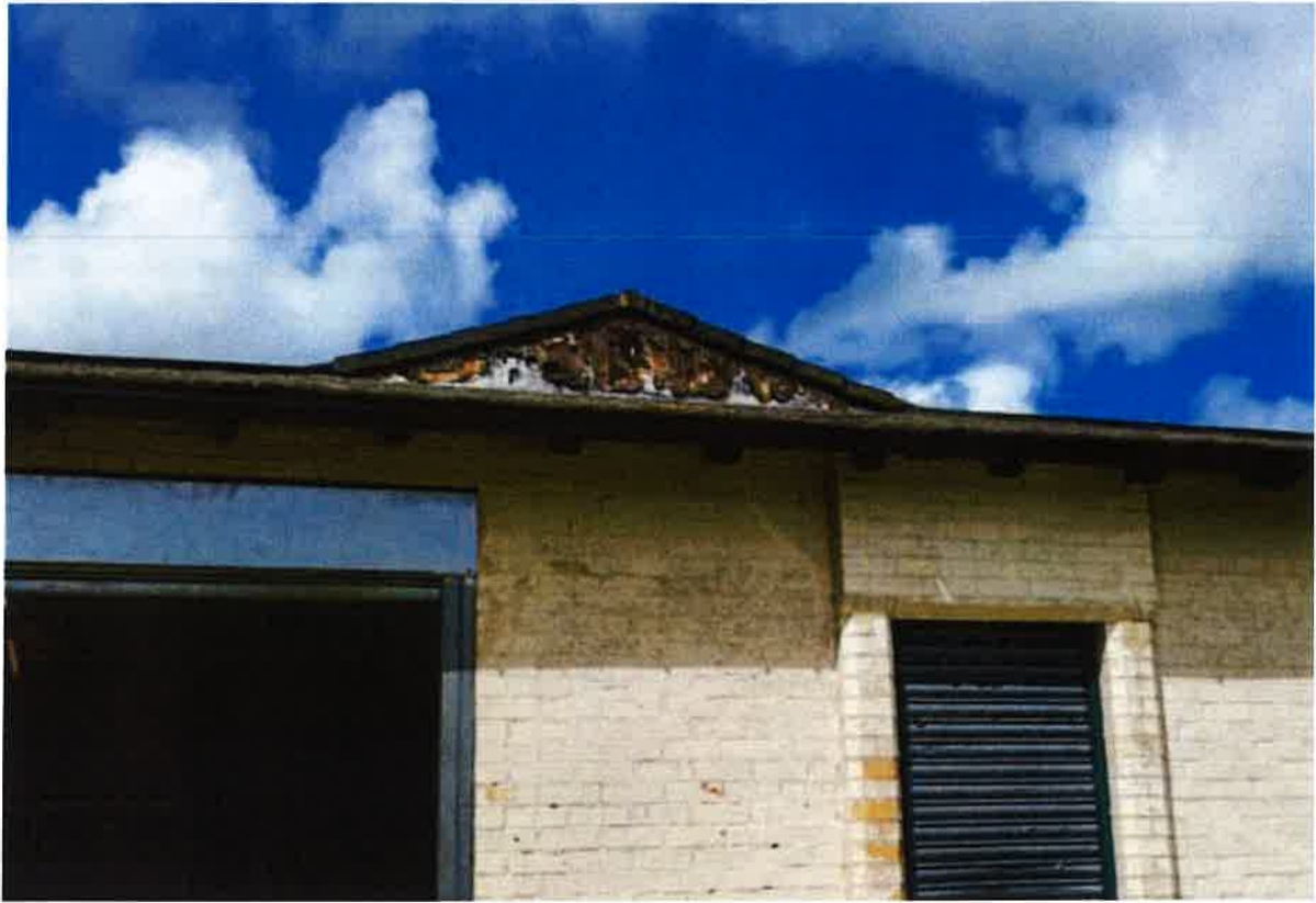
Pavilion - Roof cladding requires repair work
